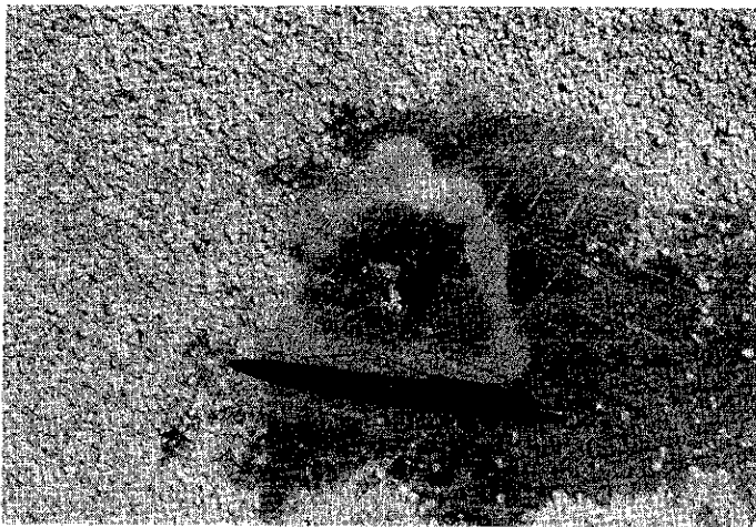
Figure 16 Mechanical Damage to Liner Under 2 ft of Sand Cover
